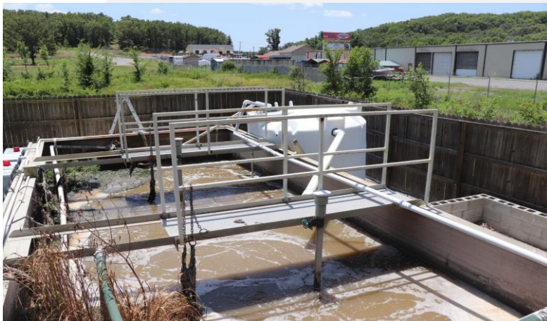
Before – Vegetation in Mechanical Plant
