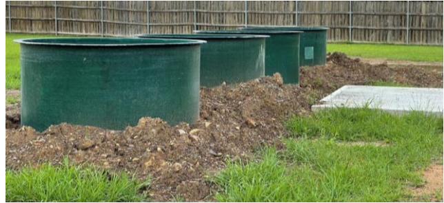
After – updated waste treatment (MBBR)
