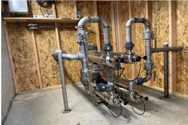
After UV Disinfection Treatment System
