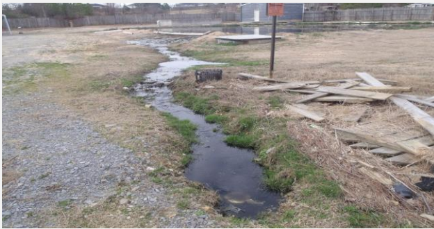
Before – Waste overflow
