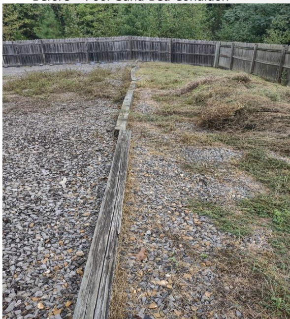
Before – Poor Sand Bed Condition
