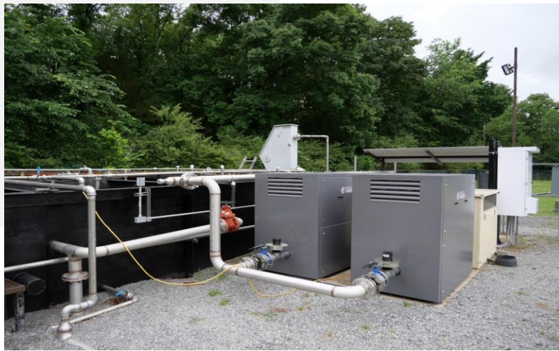
After – Upgraded facility
